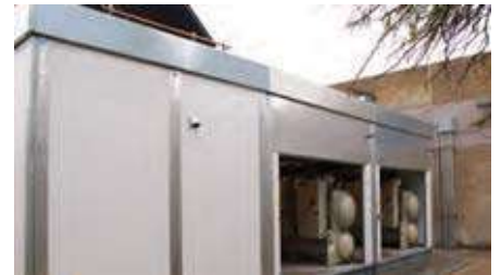
MCP with Dual Chillers Inside
