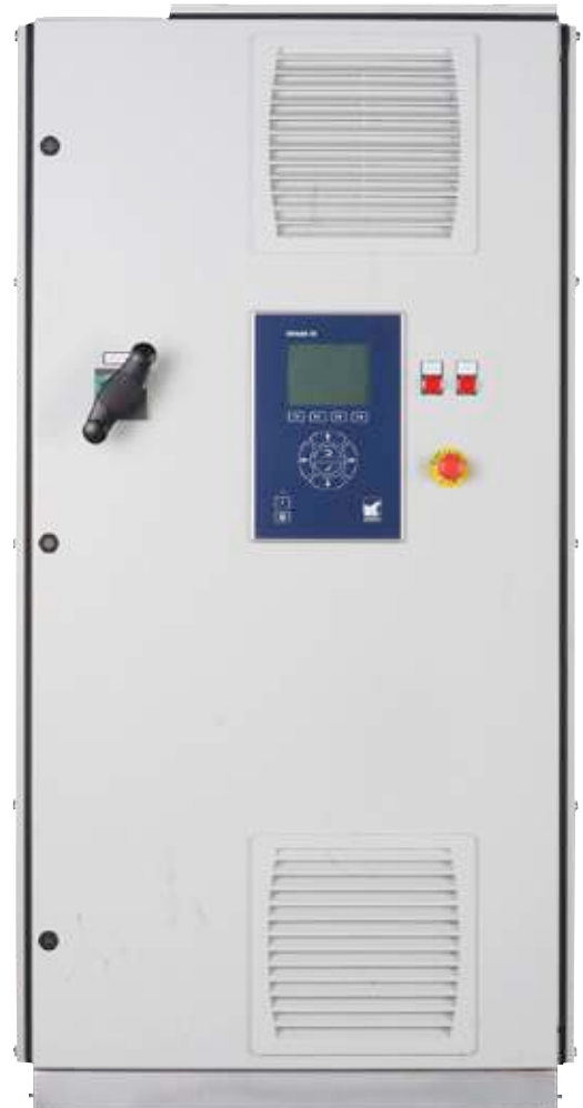
SABROE VSD panel
